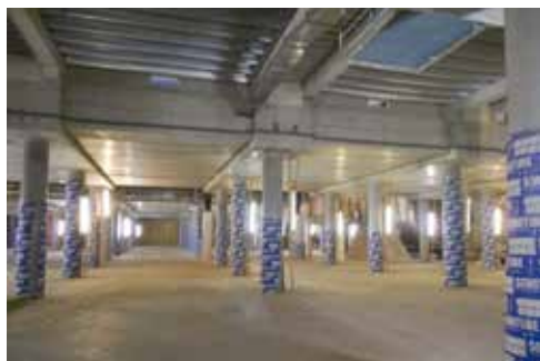
Work on the main part of the station over a period of two years between 2014 and 2015, where the station will be kept open.
