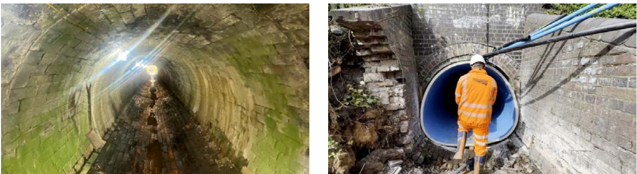
Figure 8: Upgrade a waterway culvert near Cannock to protect the Chase line in Staffordshire © Network Rail [31]
