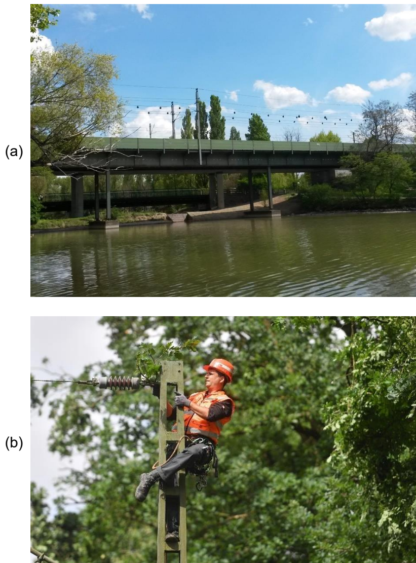
Figure 19: a) Overhead lines made visible for waterfowl to prevent collisions in a sensitive area (wetland in the city of Vienna © ÖBB-Infra, b) Vegetation trimming along the Hann. Münden, © Deutsche Bahn AG Oliver Lang
