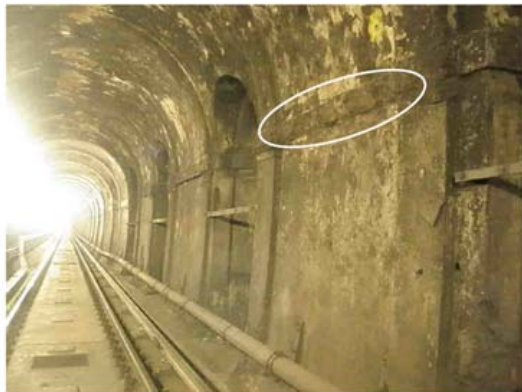
Photo 10 – Area of missing and eroded string course to Down side wall at south end.
