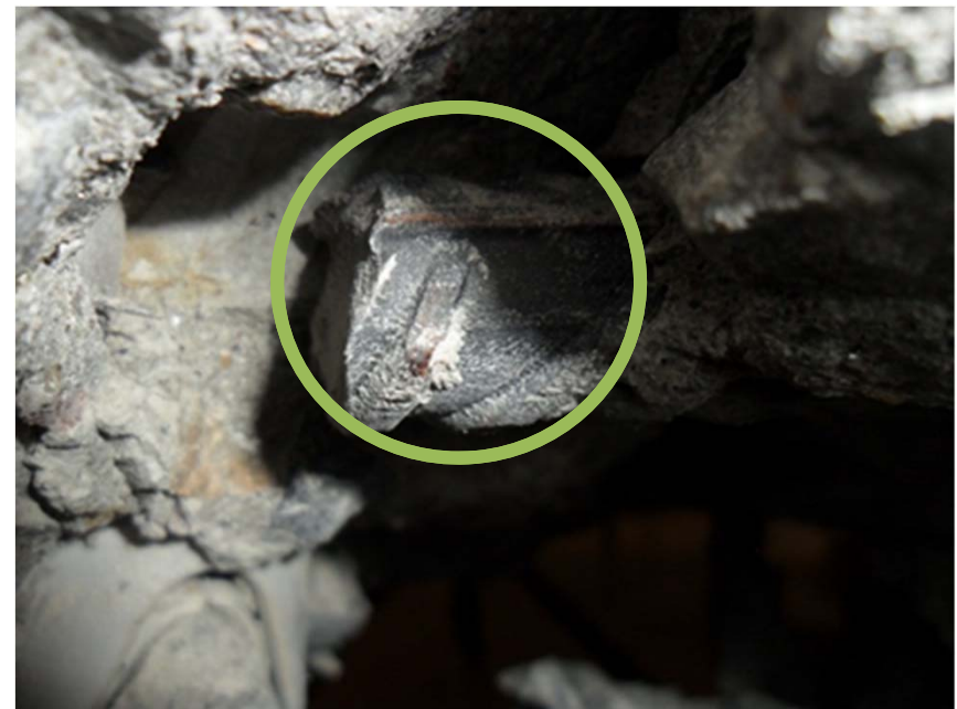
Debonding failure after rebar failed due to fatigue
